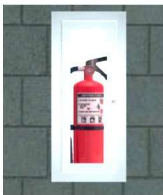
Figure 6. Fire extinguisher signage.
